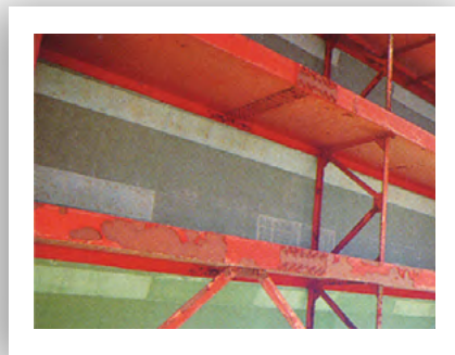
Alkyd coating is peeling
