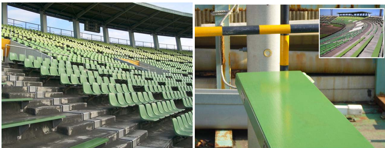
Figure 10: Fluorourethane Topcoat on FRP Stadium Seating After 20 Years
